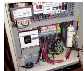
Electrical control box with built-in PLC
