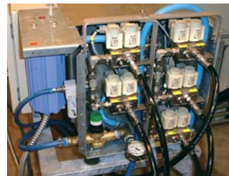
Pump unit with output valves
