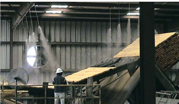
Several nozzles are mounted above the tilt hoist to knock down the fine saw dust in the air.
