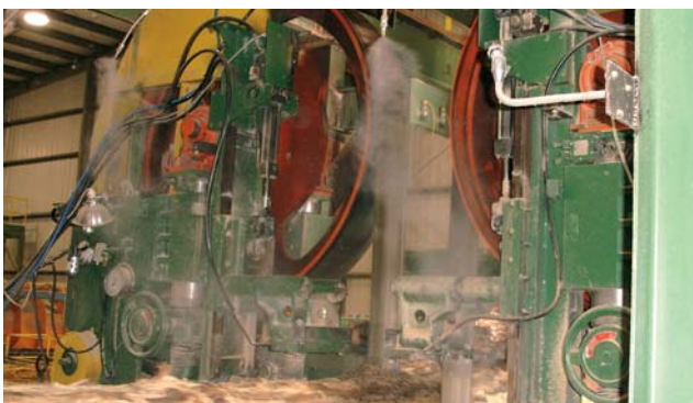
One nozzle can spray directly on the saw blade to clean and cool the saw. Additional nozzles are mounted on top of the maxi mill to knock down the fine saw dust.
