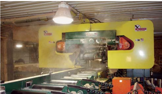
2-4 nozzles are mounted on top of the Horizontal to knock down the fine dust in the air. 1-2 nozzles spray directly on the saw blade to clean and cool the blade.
