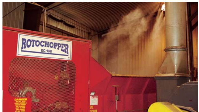
3-5 nozzles are mounted around the roto chopper to knock down the dust in the air.
