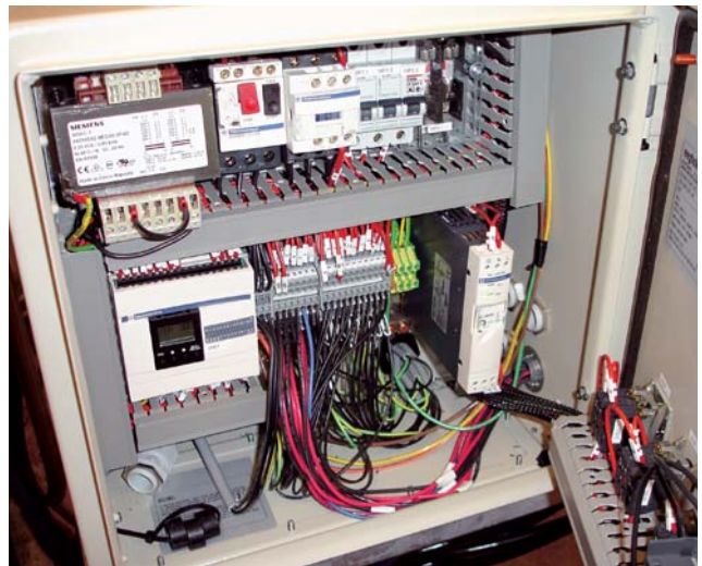
Electrical control box with built in PLC.
