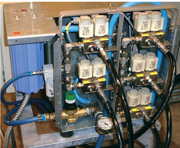
Pump unit with output valves.
